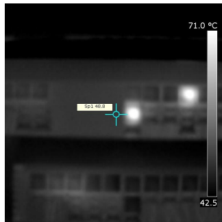
Fig. 7. Measurement of the distribution cabinet of the machine controlling part, analysis of switching elements
